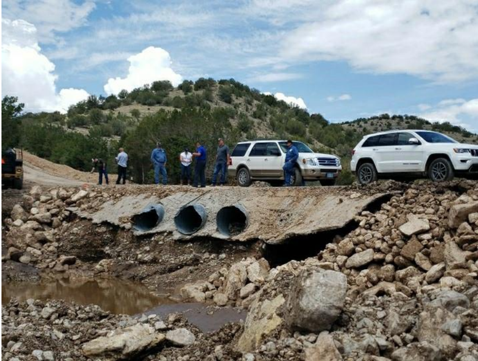
DHSEM officials examine flooding impacts on Alamo County Rd in Lincoln County
